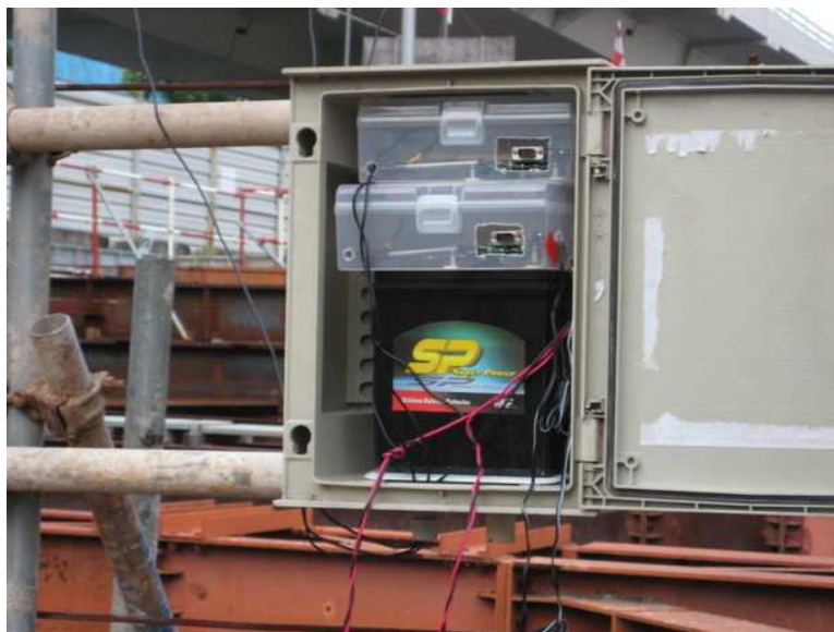
Figure 4: Base station nodes inside a box
